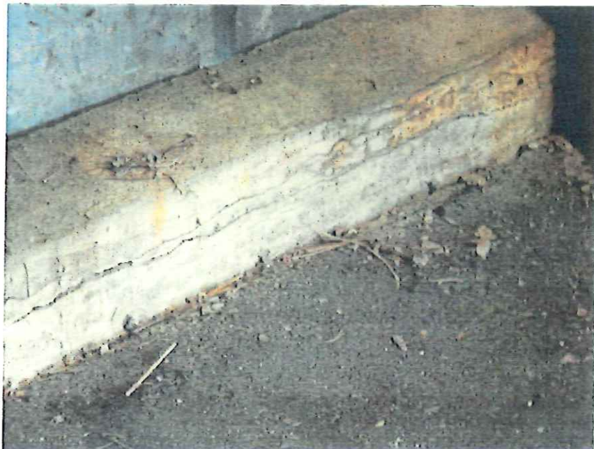
Photo 6. Foundation Wall at Northwest Corner of Building with Longitudinal Cracks
