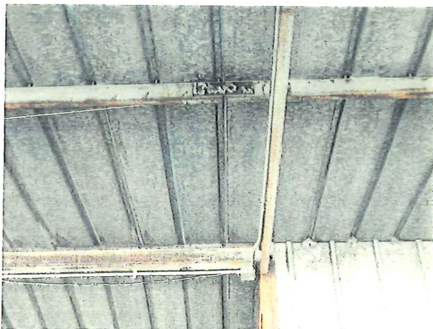
Photo 12. Typical Condition of Steel Framing with Peeling Paint and Surface Rust
