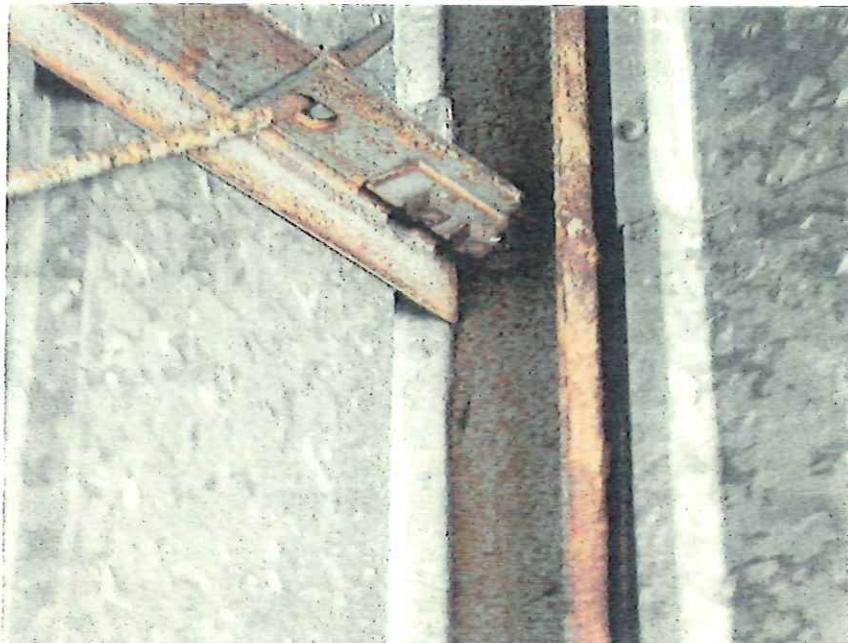
Photo 14. Typical Condition of Steel Framing at Diagonal and Horizontal Angle Connection to Steel Column
