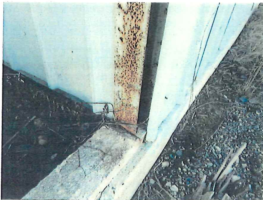
Photo 16. Exposed Steel Column at Southwest Corner of Building
