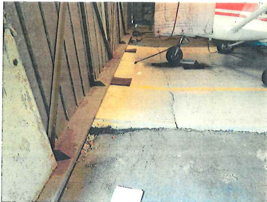
Photo 8. Pavement Settlement and Full Width Crack in Concrete Apron at Northeast Corner of Building
