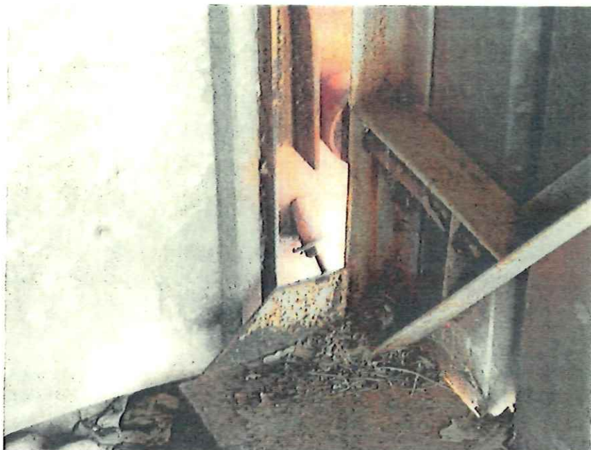
Photo 15. Typical Condition of Steel Framing at Aircraft Access Door Tracks
