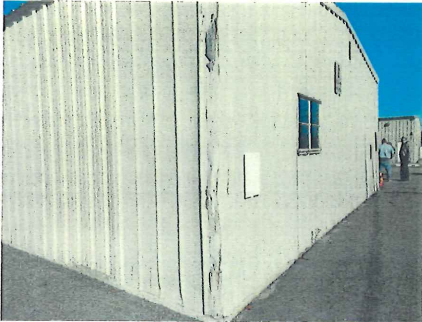
Photo 17. Damaged Metal Wall Panel and Replaced Panel Section at Southeast Corner of Building
