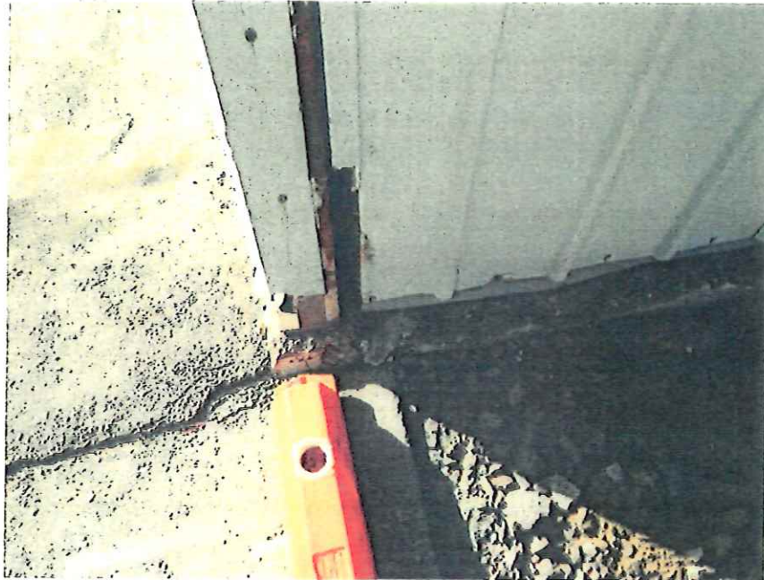
Photo 7. Concrete Spalling at Foundation Wall Adjacent Steel Column Base Plate at Northeast Corner of Building
