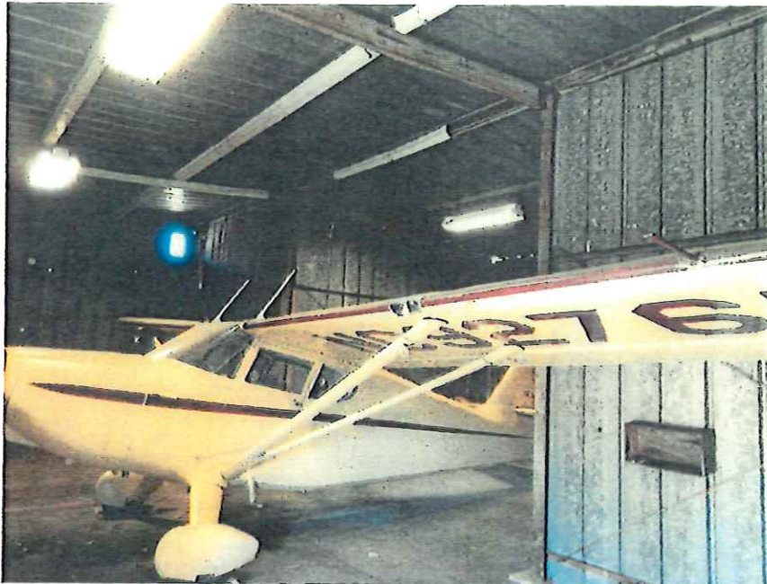
Photo 13. Typical Condition of Steel Framing with Peeling Paint and Surface Rust. Bottom of Roof Beams Covered in Aircraft Storage Room at Southwest Corner of Building
